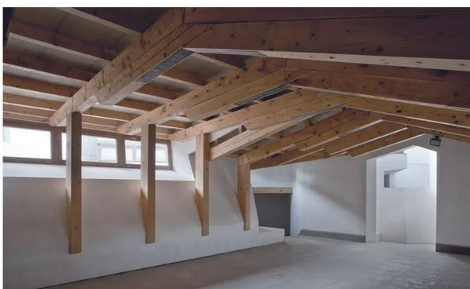
The centre will host the city's fine arts association and gallery, a museum devoted to the house itself, a public library and a roof terrace (Image credit: Adrià Goula)
